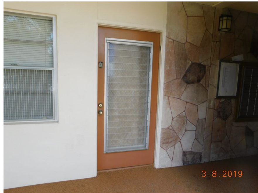
Unprotected Glazed Entry Door
