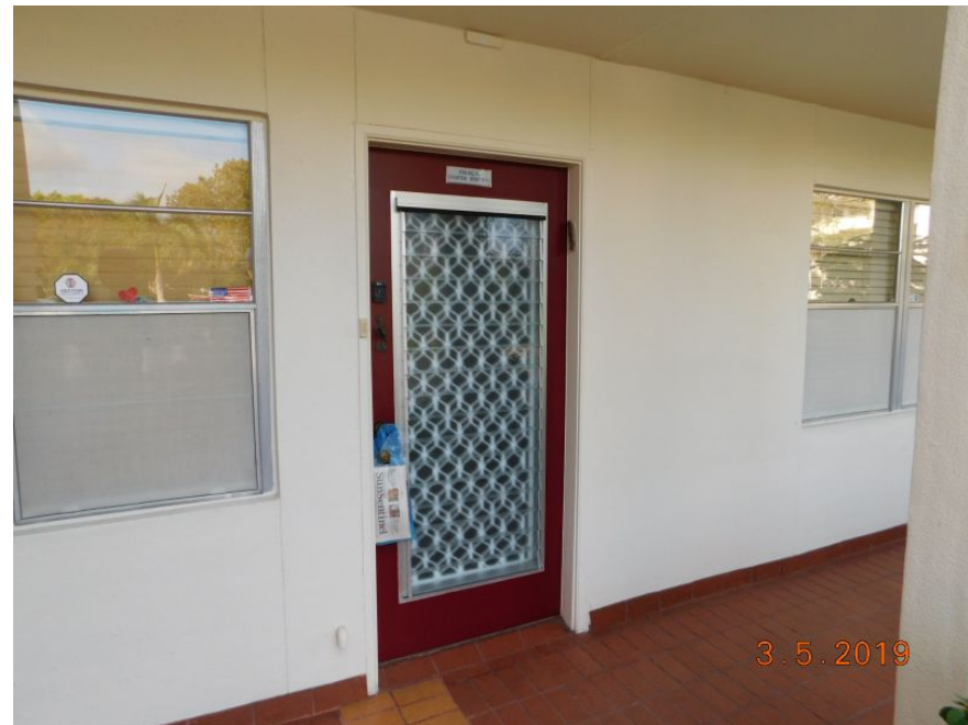
Unprotected Glazed Entry Door
