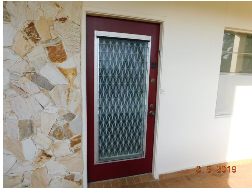
Unprotected Glazed Entry Door
