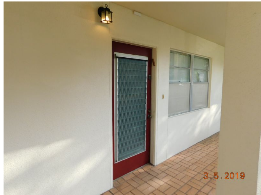
Unprotected Glazed Entry Door
