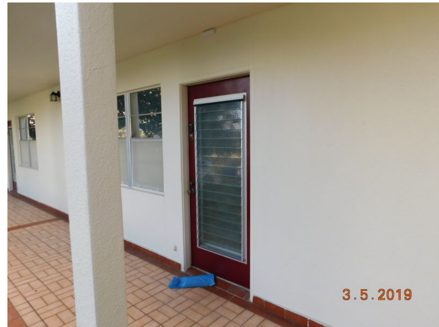
Unprotected Glazed Entry Door
