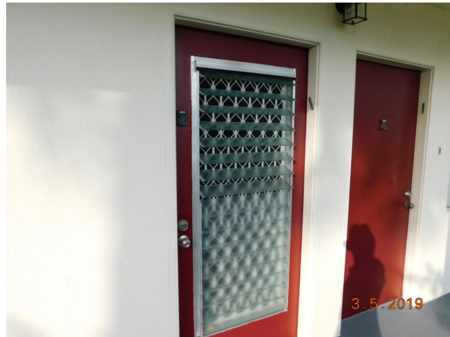
Unprotected Glazed Entry Door
