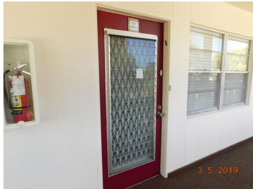
Unprotected Glazed Entry Door
