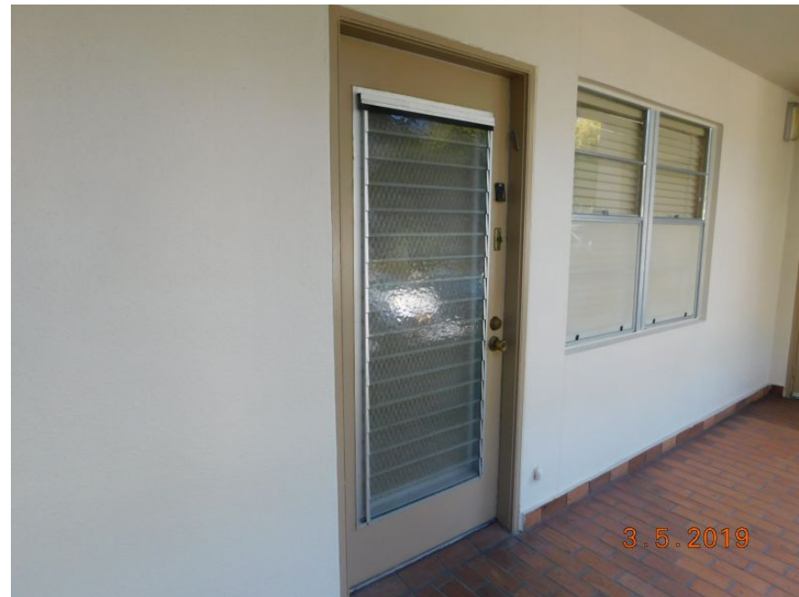
Unprotected Glazed Entry Door
