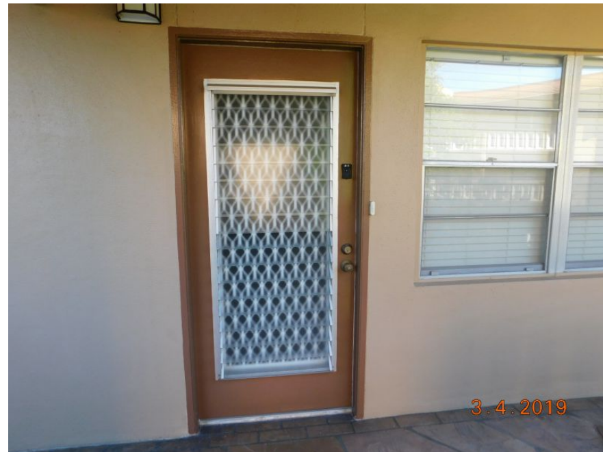
Unprotected Glazed Entry Door
