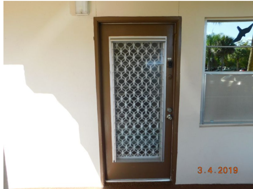
Unprotected Glazed Entry Door
