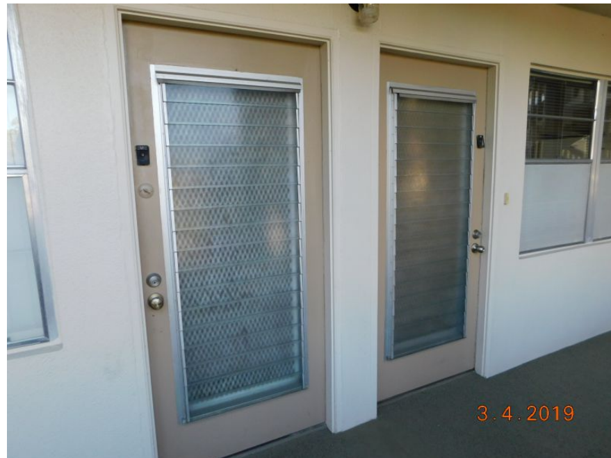
Unprotected Glazed Entry Door
