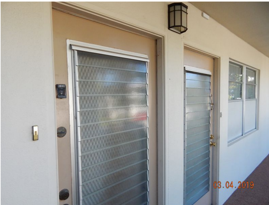
Unprotected Glazed Door
