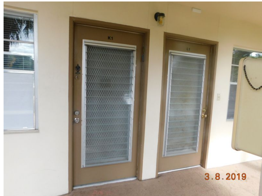
Unprotected Glazed Entry Door
