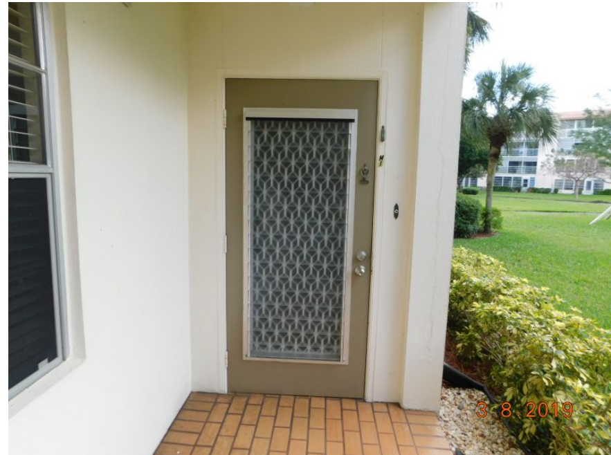
Unprotected Glazed Entry Door
