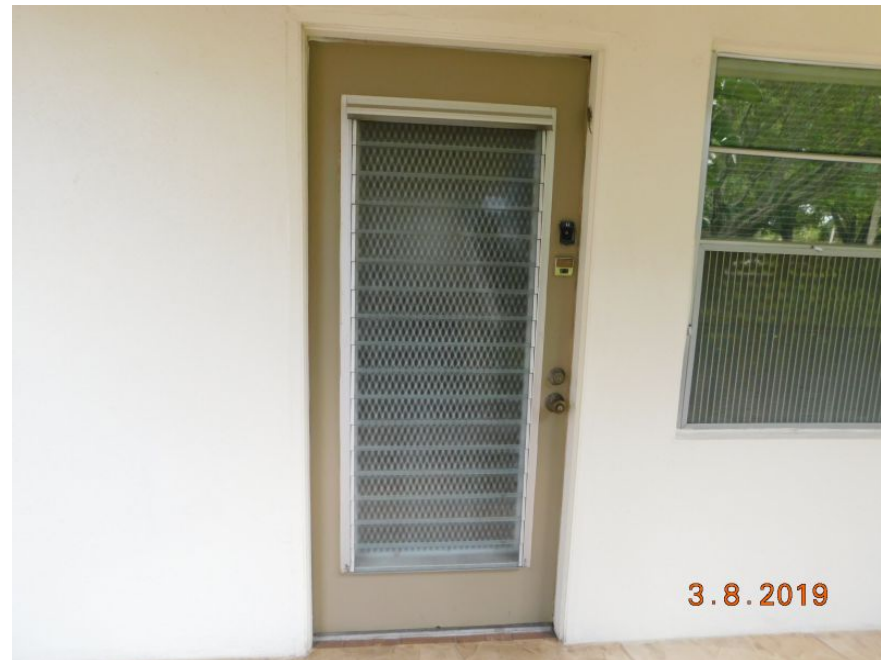
Unprotected Glazed Entry Door
