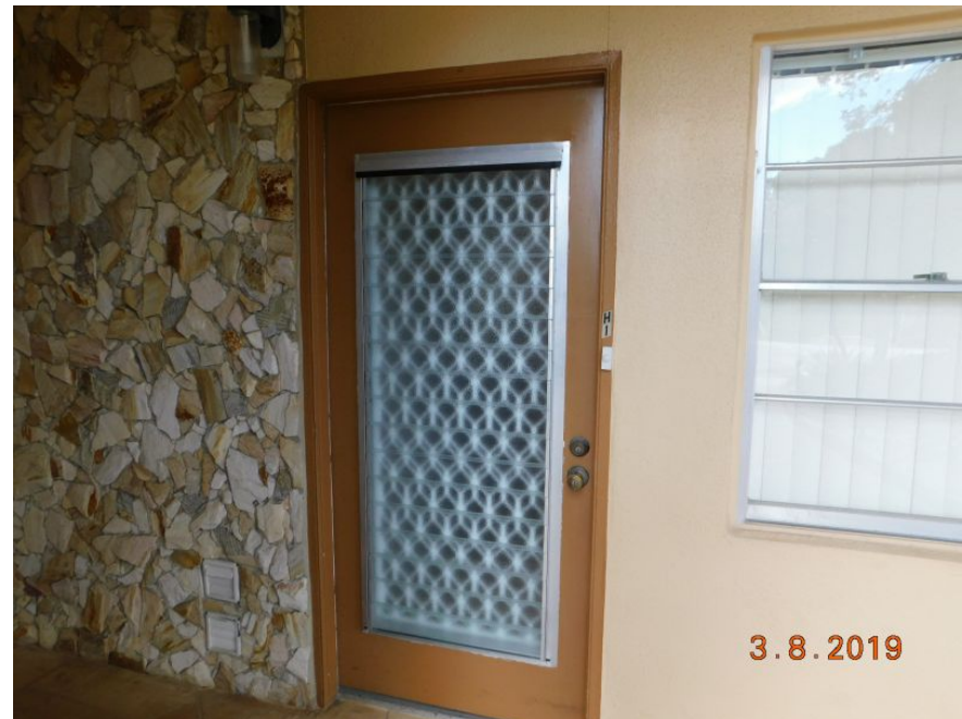
Unprotected Glazed Entry Door
