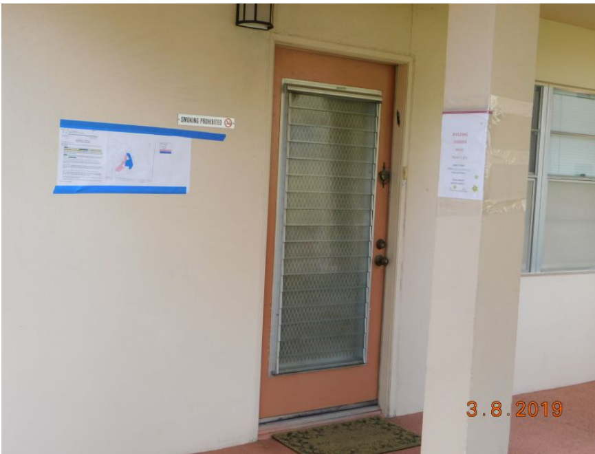
Unprotected Glazed Entry Door
