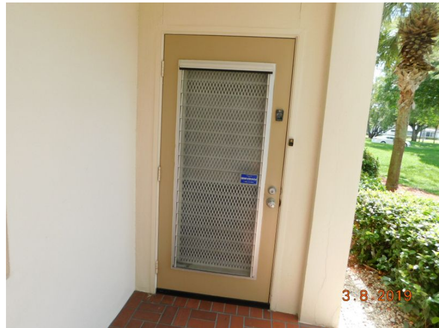
Unprotected Glazed Entry Door
