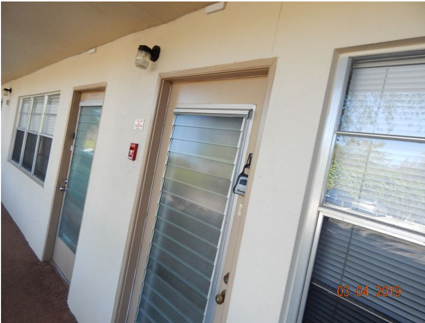
Unprotected Glazed Door
