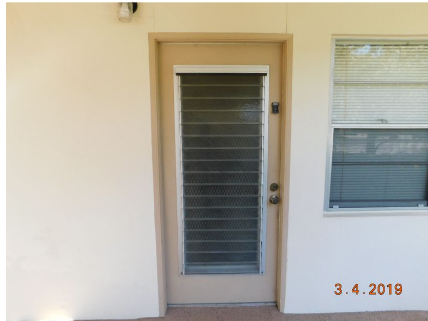
Unprotected Glazed Entry Door
