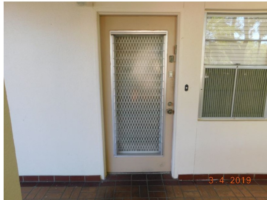
Unprotected Glazed Entry Door
