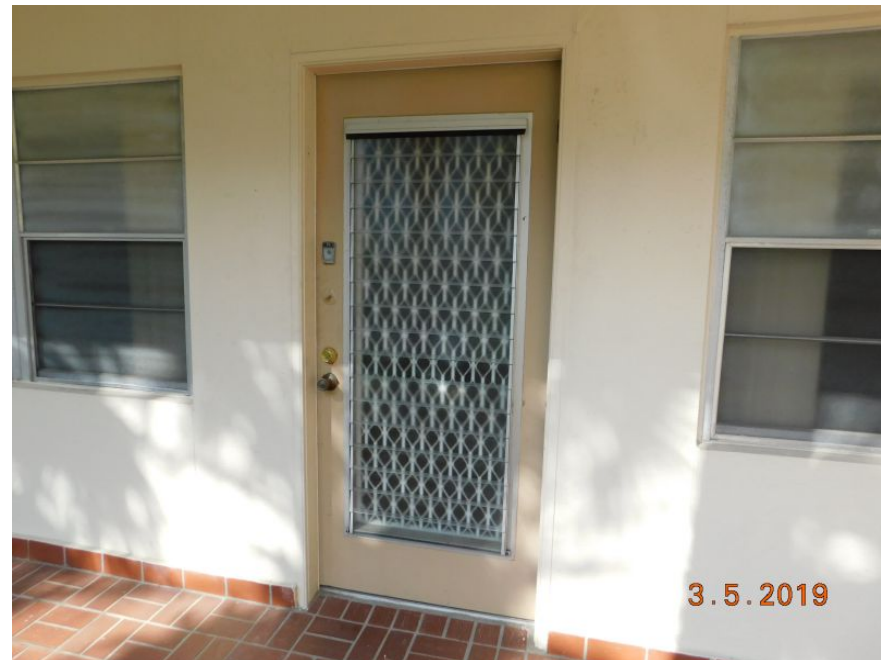
Unprotected Glazed Entry Door
