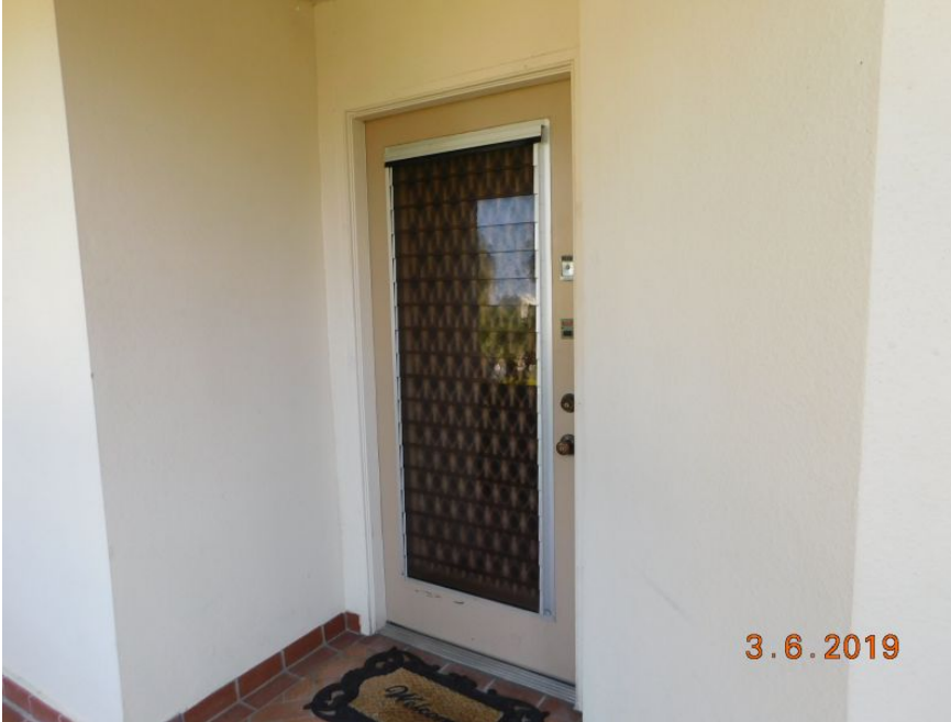
Unprotected Glazed Entry Door
