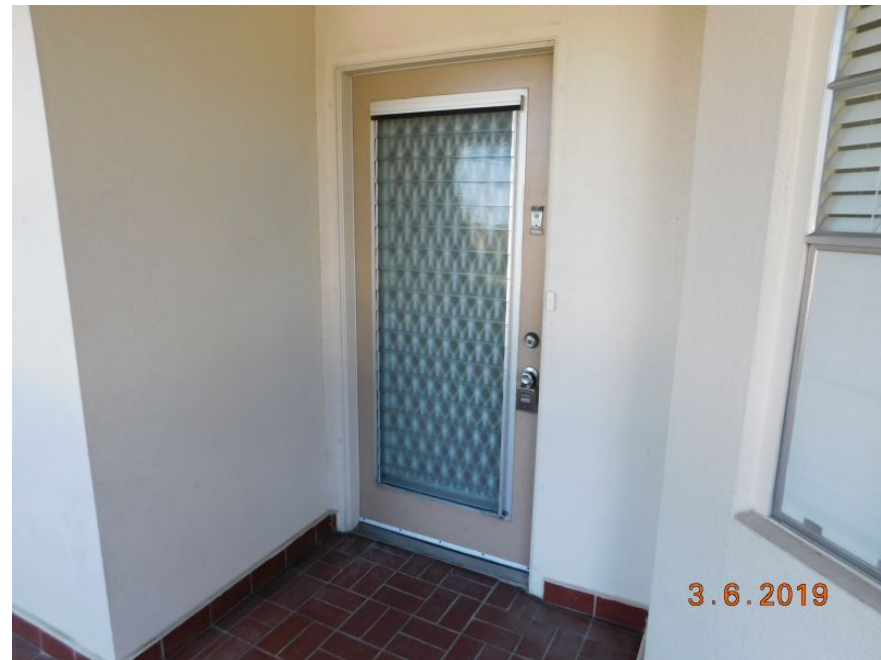
Unprotected Glazed Entry Door
